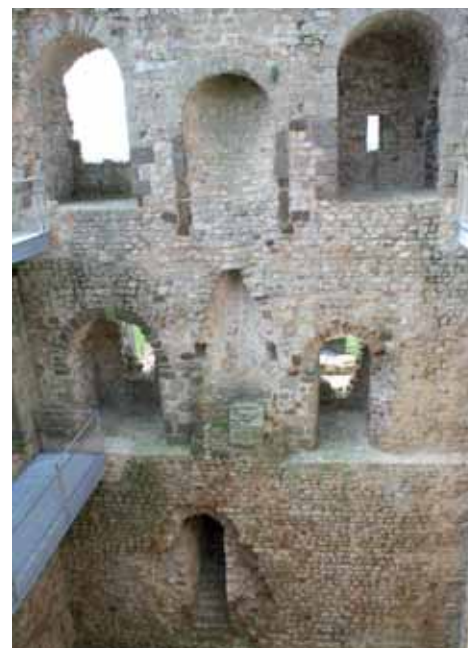
Inner of the keep, south-west wall. The arches at the centre of the 1 st and the 2 nd floor are the remnants of the filled in again chimneys.
